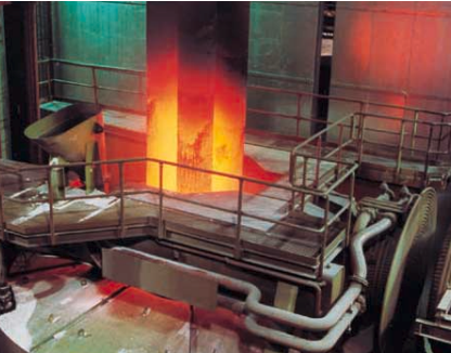
140-t UHP electric arc furnace
