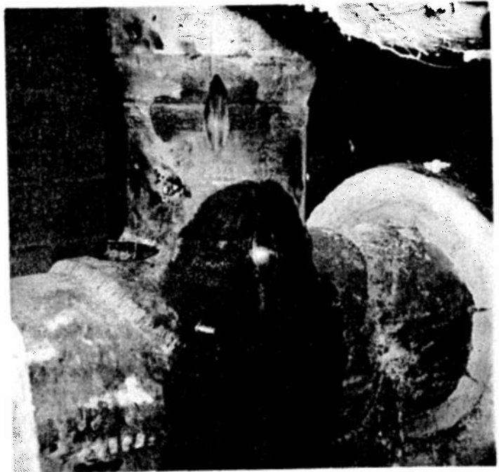
Fig. 4. Appearance of piping after removal of boat-shaped weld-probe specimen from pipe-to-valve and pipe-to-saddle joints.
