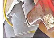
These large galvanized sections, have all been 'cope cracked' in the c
