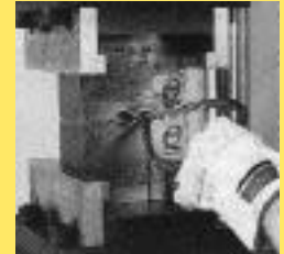
The sleeve is pressed onto the splice end. This cold forming process lets the soft sleeve metal flow into all rope gaps.
