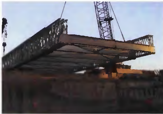
A crane lifts a temporary steel bridge leased from Acrow Corp. onto its abutments for the southbound lanes of Interstate 95. Crews quickly installed the steel deck panels and added an asphalt wearing layer in order to restore traffic. (Photo courtesy of Acrow Corp.)
