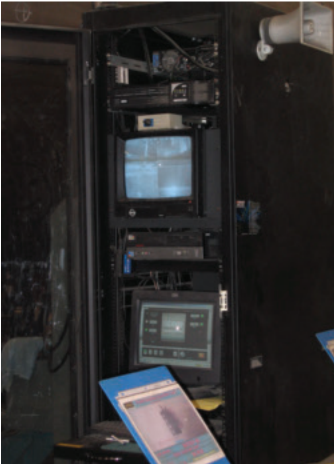
Fig. 8 — The closed-circuit television system used to monitor employees working inside a tank, which is considered a confined space.
