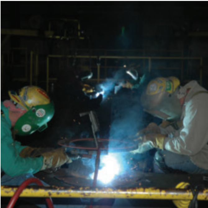
Fig. 10 — These workers are welding nozzles and repads into the tank car. The weld requires complete joint penetration with ultrasonic NDE requirements, using FCAW. Note the safety harnesses, which are connected to the access platform for fall protection.
