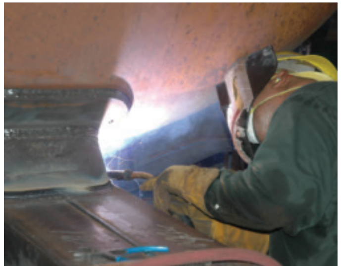
Fig. 6 — Using the FCAW process, a welder works on a head shoe. The head shoe is the reinforcement between the tank and the stub sill, which is the device that connects two rail cars.
