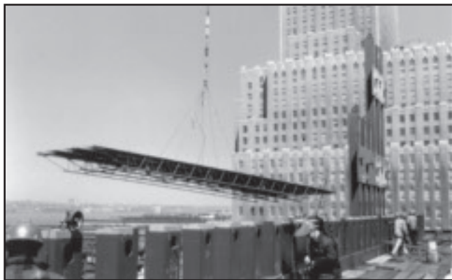
Fig. 2 — Undated construction photograph of a composite floor assembly being hoisted into place.
