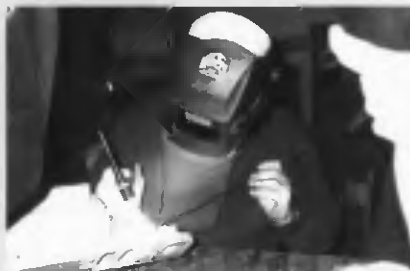
Jerry Doherty demonstrating the proper technique of repair welding on cast iron at the second session of the Reading Section's Welding Seminar.
