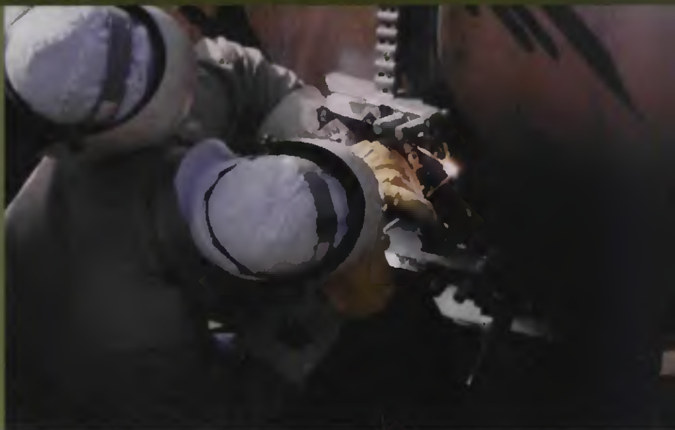
Chain clamp is used to align and hold in position 48-in. pipe for welding.
