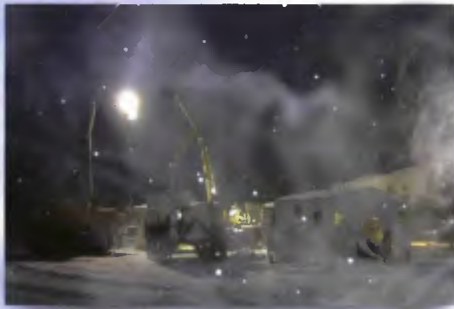
Welders work in near-arctic conditions on a section of a TransCanada gas pipeline using X120 linepipe.
