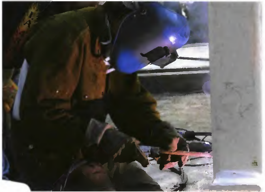
Fig. 1 — Fabrication of the trusses was on a fast track in order to meet the philharmonic's summer concert schedule.
