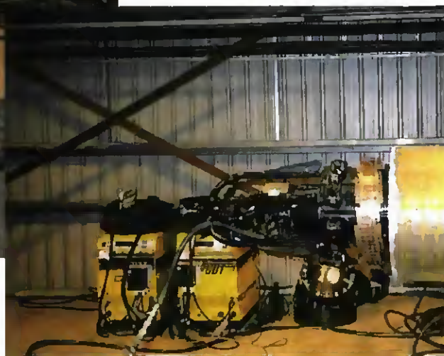
Fig. 2 — An internal clamp with backing shoes is used for the root run.
