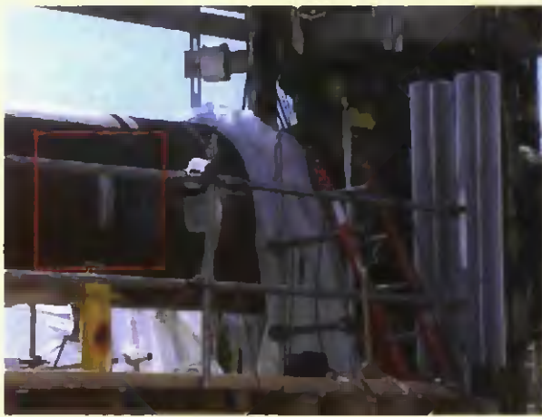
Fig. 8 — Fitting material welded to pipe material adjacent to RGV prior to removal.
