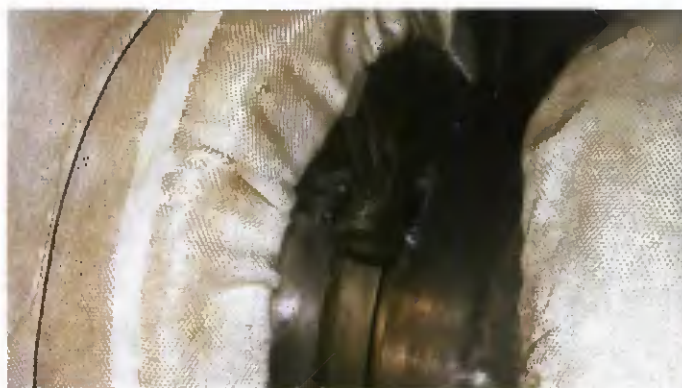
Fig. 4 — Fitup and alignment were maintained by using a section of P91 pipe with a carbon-steel handle.
