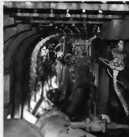
Learning well the hard way, a Triangle student effects welded repairs according to code and a well-planned procedure.
