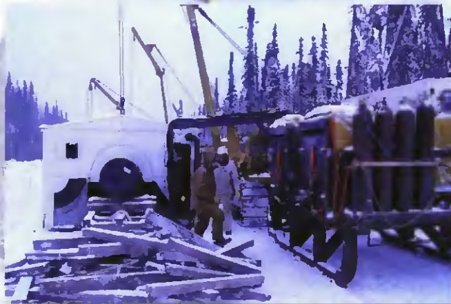
Welding equipment sleds (right) were pulled by tractors. Welding sheds (left) were lowered over pipe ends by cranes.
