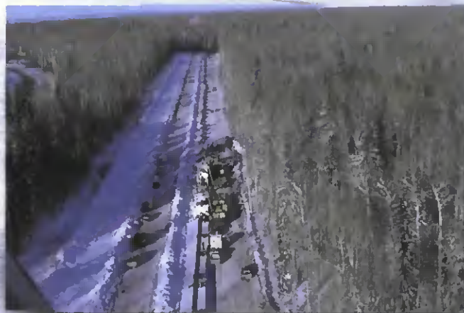
Aerial view of the X120 pipe laying operation, showing the array of heavy equipment needed.
