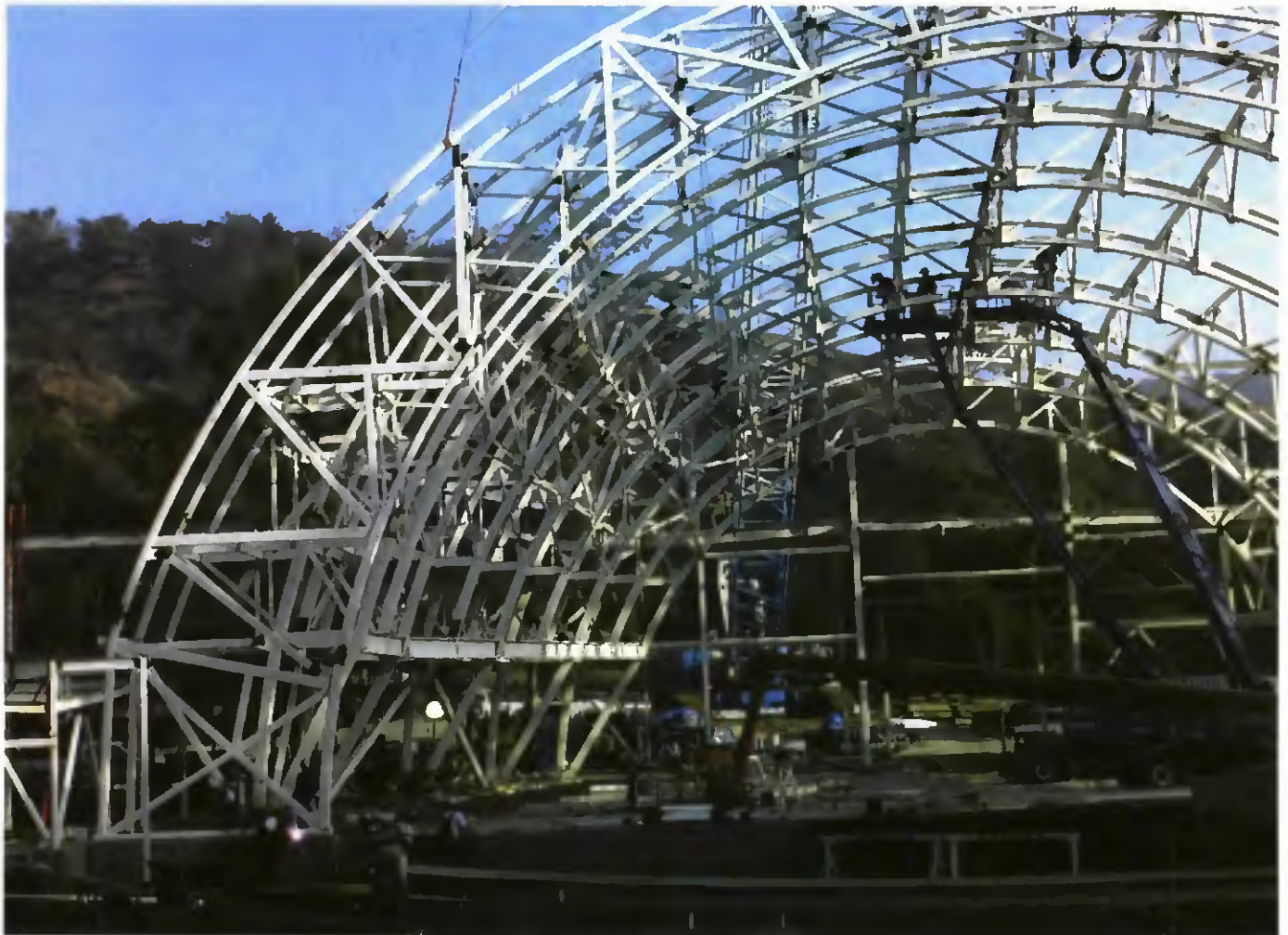
Fig. 2 — Much of the field welding took place at heights 42 ft or more from the ground.
